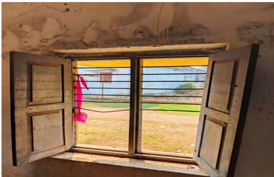
Figure 4: Broken window of Anganwadi Center by Sloth Bear.
