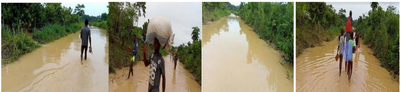
Figure 6. Poor nature of road that links Asankrangwa and Affiena.
